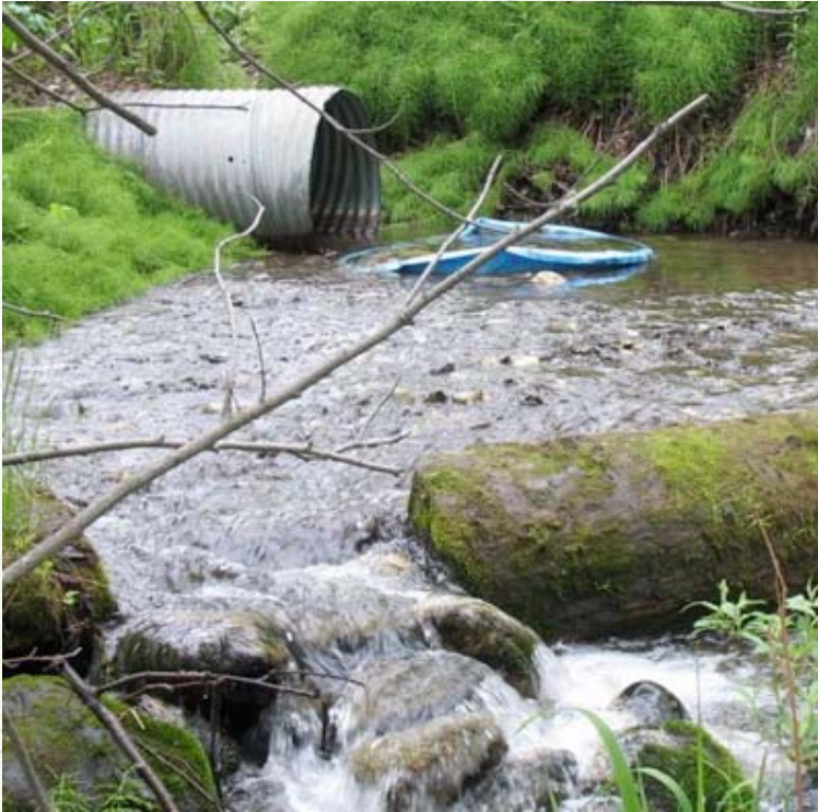
Incorrect Pool idea.
